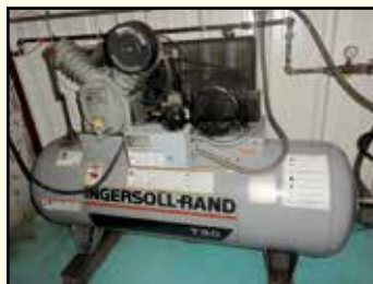
< INGERSOLL RAND Air Compressor, Mdl. T-30, horizontal, 5 HP, SN 00030753.
